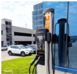
ChargePoint CT4000 EV charging station at a workplace
